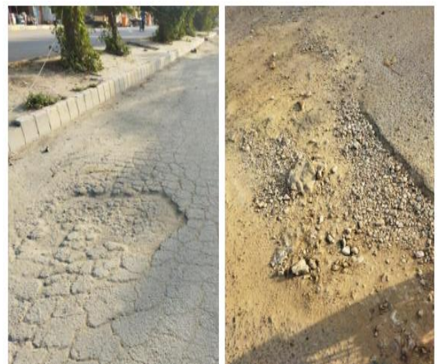
Fig. 1. Dilapidated Roads in Karachi (Alligator and Patching)
