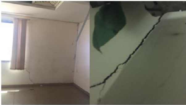
Fig. 2. Shows cracked wall at one of university buildings
