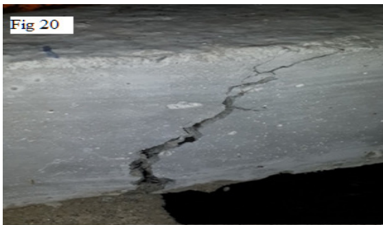
Fig. 20: Failure of slab S3 (5.0 %) in Flexure
