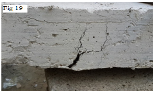
Fig. 19: Failure of slab S2 (2.5% MD) in flexure and shear
