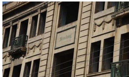
Damaged details of surface decoration
