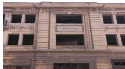
Dirt accumulated and soiled façade
