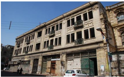
Ground floor showing signs of wearing
