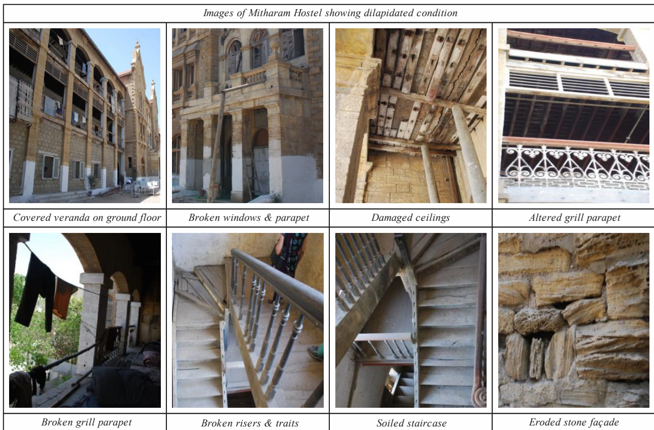
FIG. 11. IMAGES OF MITHARAM HOSTEL SHOWING DILAPIDATED STATE
