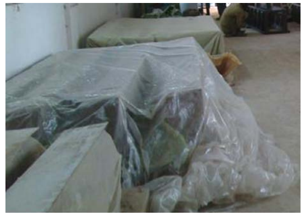
FIG. 4. LOAM MASONRY WALL UNITS COVERED WITH PLASTIC SHEET ARE BEING DRIED IN SHADE
