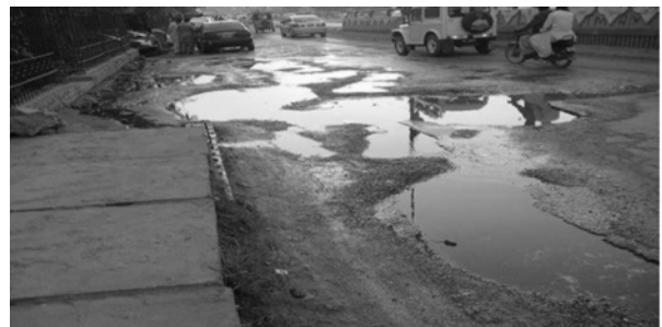
FIG. 2. POOR CONDITION OF ROAD IN QASIMABAD
