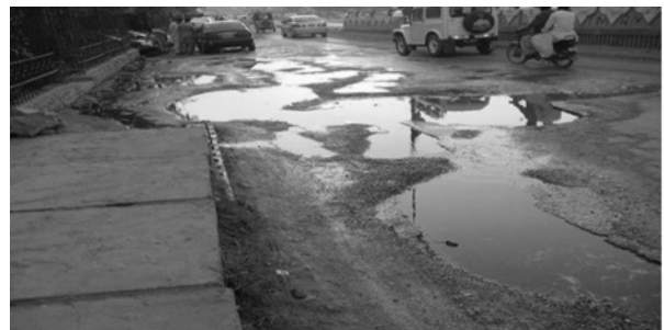
FIG. 2. POOR CONDITION OF ROAD IN QASIMABAD
