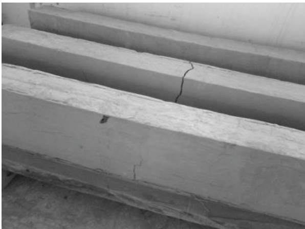
FIG. 6. DRYING CRACKS IN BASE OF THE CLAY BEAM
