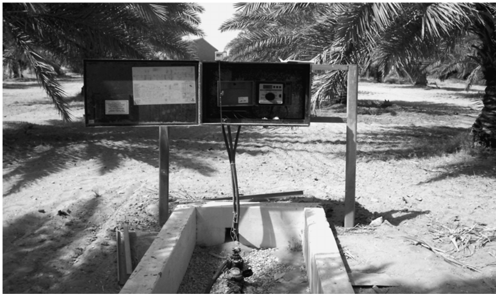
FIG. 3. TOTAL CENTRAL CONTROL PANEL
